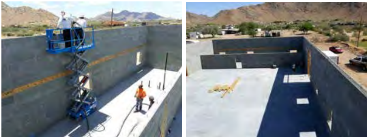
OSB buck with anchor bolts at mid height on an ICCF wall.
