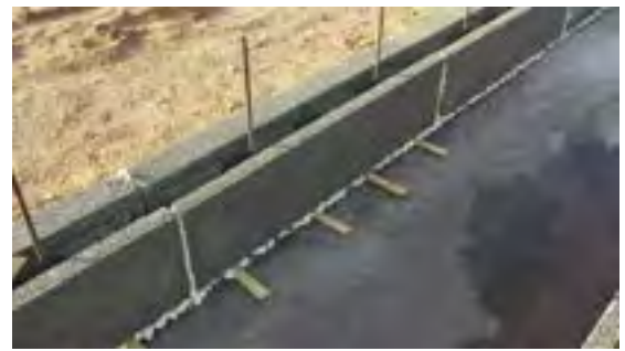
Photo 7.6c Plumb and level and polyurethane foam adhesive in place. Take great care not to move the block when tacking block in place. 15 to 20 minutes later, when the tack gluing dries, you can "super glue" (glue every 3-4") the block.
