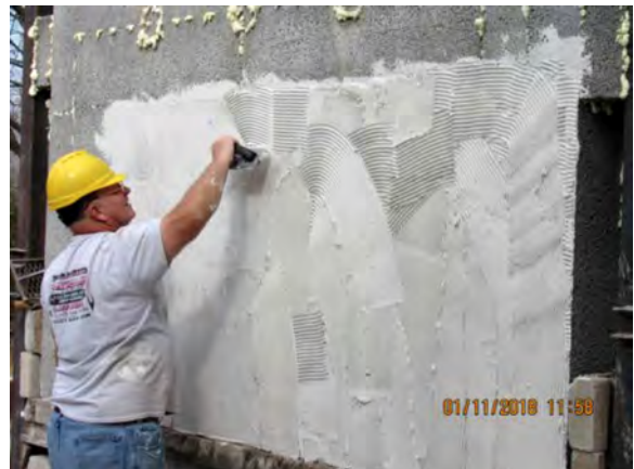
You can fully mud the wall or the back of the board
